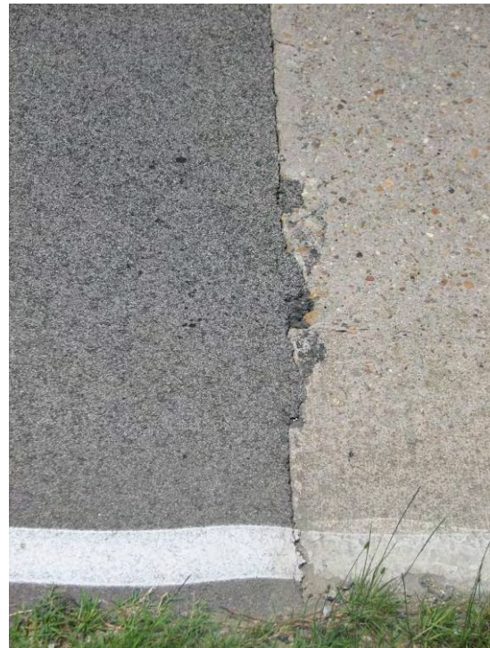
Tight joints have been maintained, material has not bled, or streaked away from the patch
